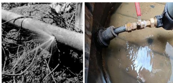
Slika 2.2. Curenje na opskrbnom cjevovodu (uličnom vodu) lijevo i kućnom priključku desno (Losses in Water Distribution Networks – A Practitioner’s Guide to Assessment, Monitoring and Control, Malcolm Farley and Stuart Trow, IWA Publishing, 2003)
